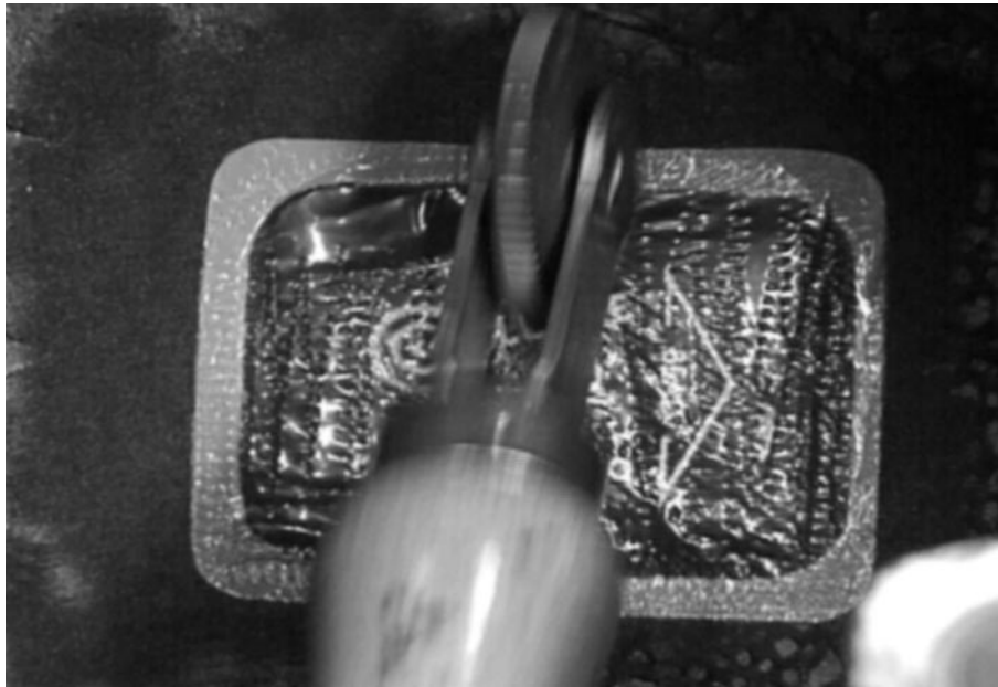
Using a stitching tool to remove trapped air and seal the edges of the repair unit.
