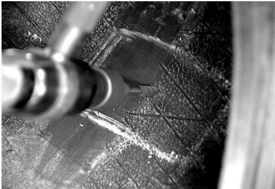
A carbide cutter mounted to a low-speed drill is used to remove the frayed ends of damaged steel cords.
